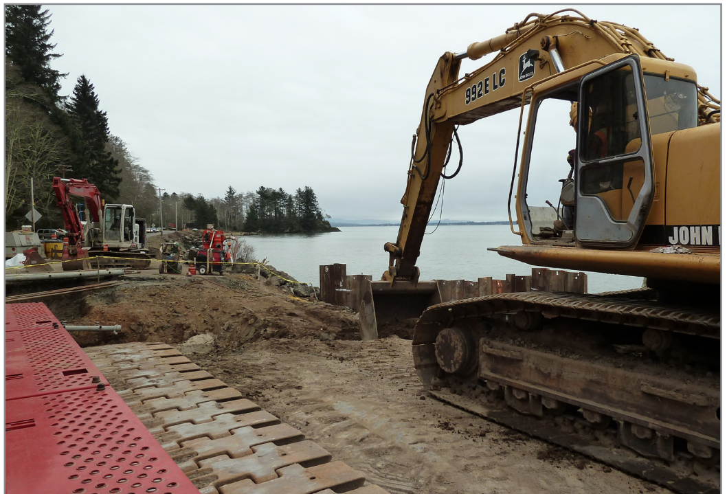
Construction crews prepare channel for culvert that will re-open historic tidal wetlands in the Columbia River estuary.
